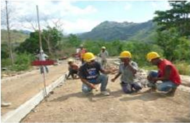
Fig. 9 Setting out and placement of formwork (Source: Manual Pavement-Labour Based Technology for Rural Road Works)
