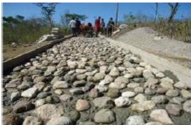
Fig. 10 Placing of Plums on Lean Concrete (Source: Manual Pavement-Labour Based Technology for Rural Road Works)
