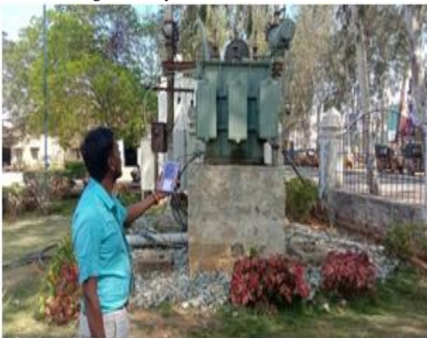
Fig. 6 Testing of Live Wire condition with proposed model (Venue: Kuppam Engineering College Campus)
