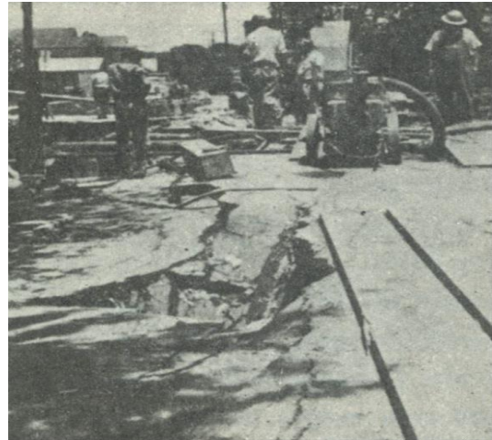
Fig. 1. Pavement subsidence after damage on the old water supply system in the city of Mobile, Alabama, USA [9].
