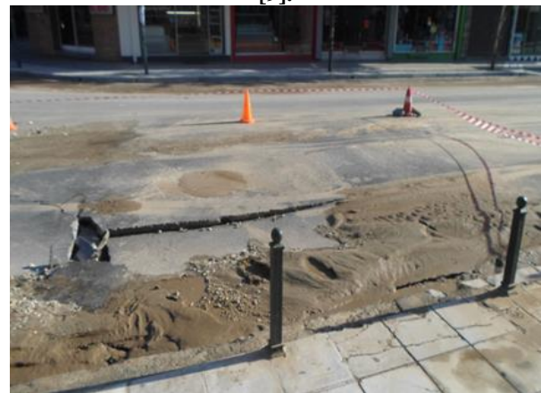
Fig. 2. Pavement destruction due to corrosion of the water pipe, Cyprus Street, Larissa.
