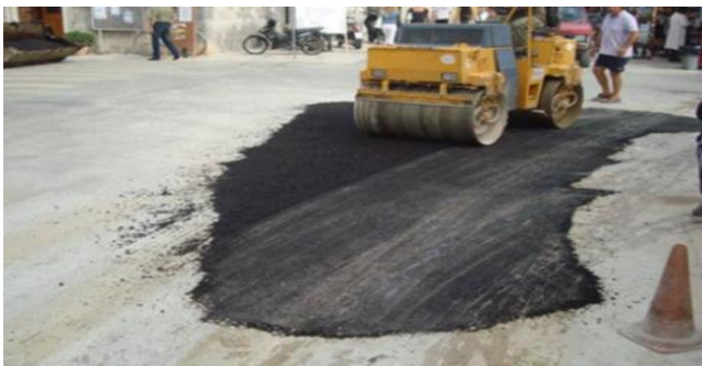
Fig. 4. Compaction of asphalt mix by vibratory roller following water supply network failure.
