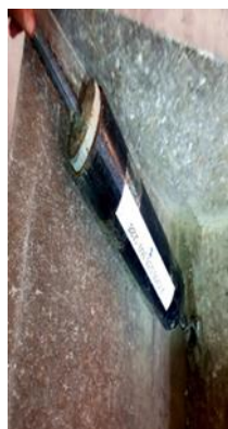
Fig. 10 Grout to sleeve bond failure
