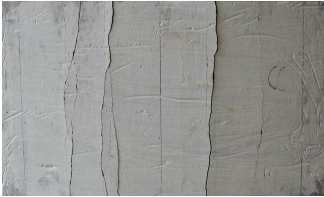
Fig. 24 Crack pattern of single layer crimped panel
