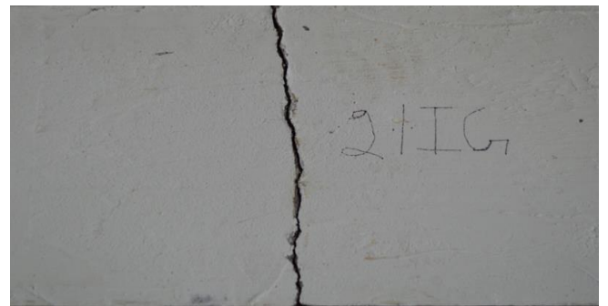
Fig. 18 crack pattern for 2% inhibited single layer galvanized panel
