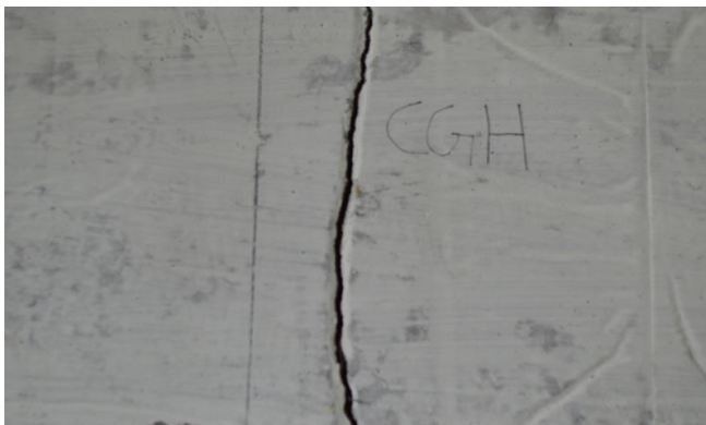
Fig.20 Crack pattern of single layer galvanized panel
