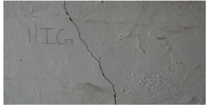
Fig. 17 crack pattern of 1% inhibited single layer galvanized panel
