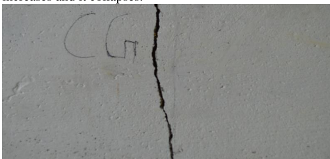
Fig.16 Crack pattern of single layer galvanized panel
