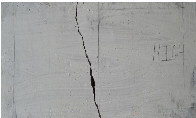
Fig.21 Crack pattern of 1% inhibited single layer galvanized panel
