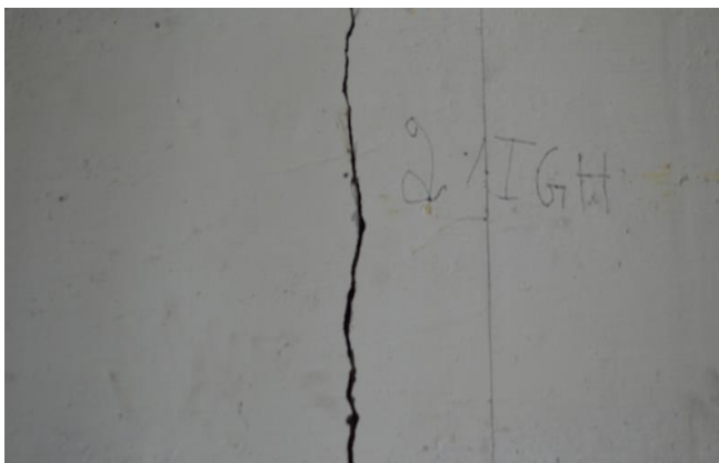
Fig.22 Crack pattern of 2% inhibited single layer galvanized panel
