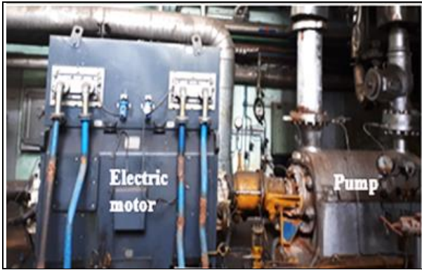
Fig. 2. Photo of Boiler feed pump Thermal Power plant
