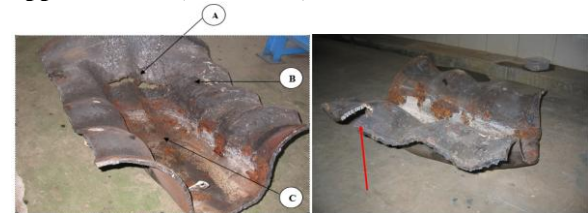
Figure 9. Furnace - the upper waterside that has failed, shows a change in shape (plastic deformation). A, B and C are the test sample areas.
