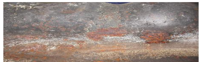
Figure 11. Fractography of a furnace - the upper waterside at Location B
