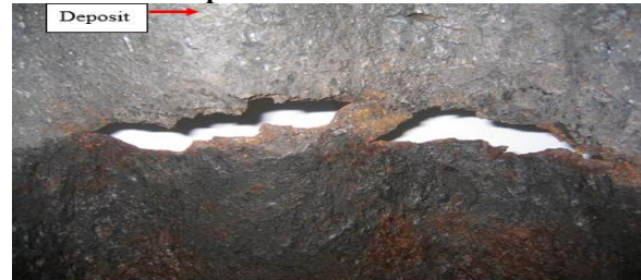
Figure 10. Fractography of the furnace wall - the upper waterside at Location A
