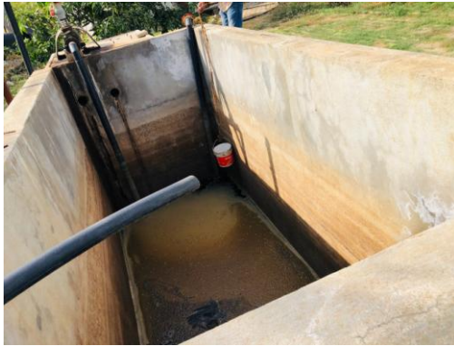
Figure 1 Landfill leachate collection tank
