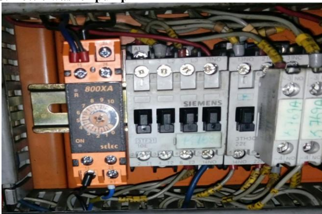
Figure 7: Secondary Pump -II
