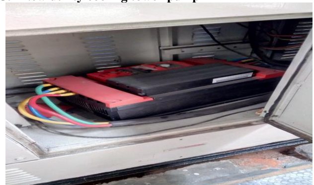
Figure 4: Cooling Tower Pump
