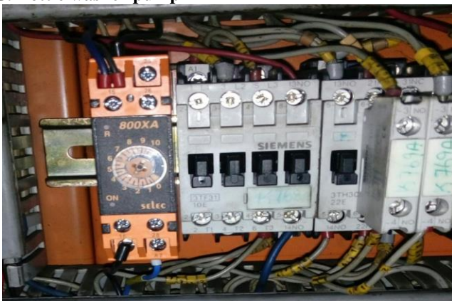
Figure 7: Secondary Pump -II
