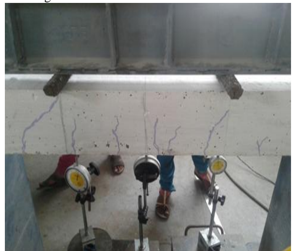
Fig 1 Crack formation in the RC Beam
