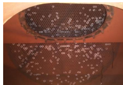
Figure – 9 Identified punctured tubes
