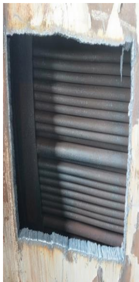
Figure – 12 Feed water Heater Tube Bundles
