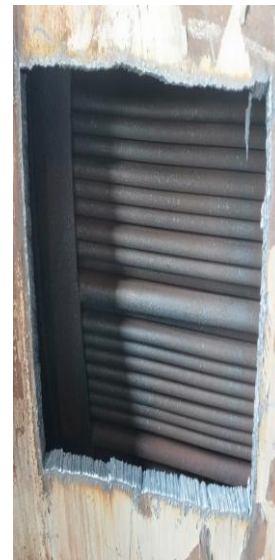
Figure – 12 Feed water Heater Tube Bundles
