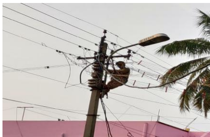
Fig 1.1 Line man working in the post
