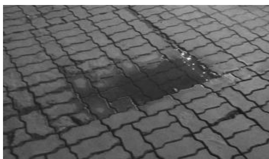
Fig. 2 ICBP pavement with depression and accumulated water in the depressed area
