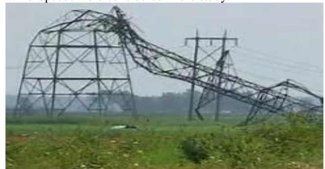
Figure 1: Collapse Of Transmission Line Tower
