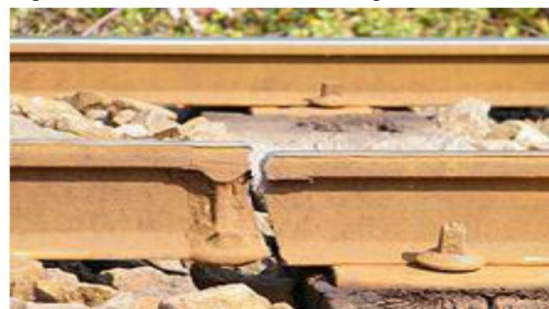
Fig 1: Railway Track Crack
