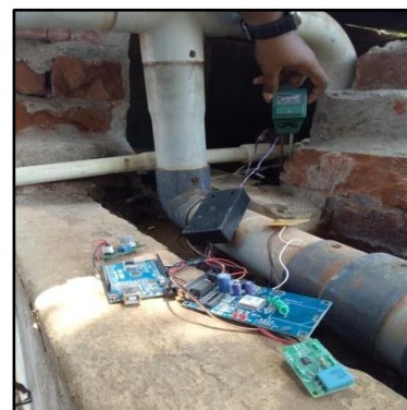
Fig 3: Real time water quality Monitoring from the sump
