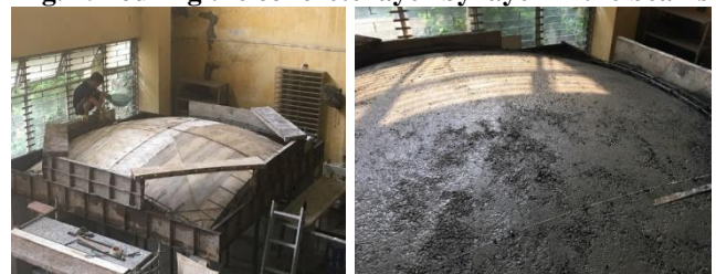
Fig. 5. Creating formwork and pouring the concrete layer by layer in the shell
