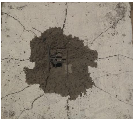
Fig 8(C): Crack pattern for GC2 slab
