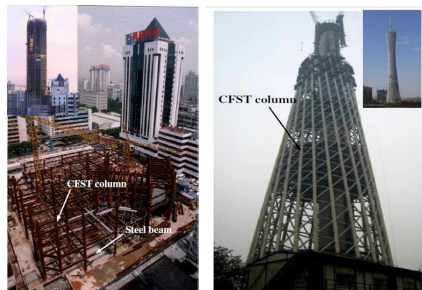
(a) SEG Plaza in Shenzhen (b) Canton Tower in Guangzhou
