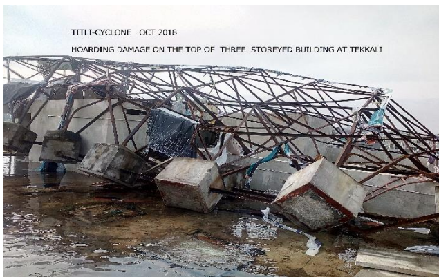
Fig 1. Hoarding damage in Titly cyclone-2018
