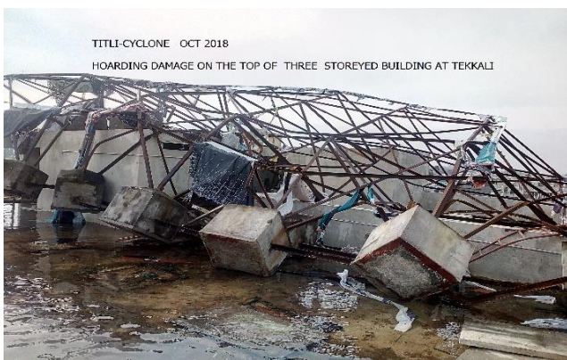
Fig 1. Hoarding damage in Titly cyclone-2018
