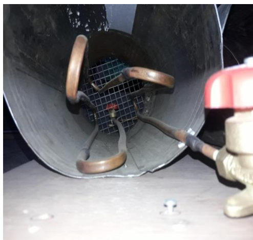
Fig. 4: Condensers tubes are placed in the shell
