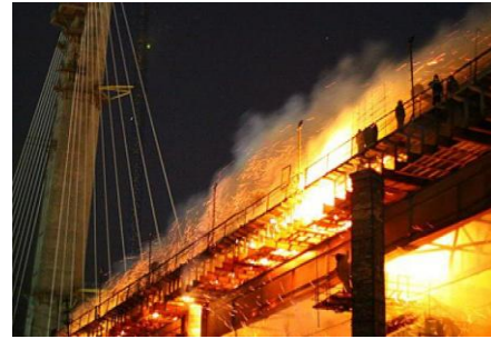
Fig. 1. Bridge constructed over ZolotoiRog Bay caught fire
