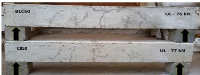
Fig 4. Crack pattern of CB50 and BLC50 beams
