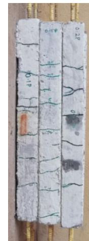
Fig 11. Crack pattern of polypropylene fibre reinforced UHPC
