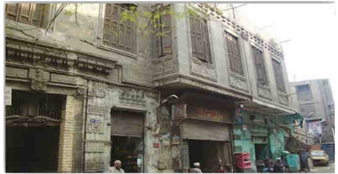
Figure (3) very old building which reflects neglecting the periodic maintenance work (Amani Elsaied Abdulrahman Ahmed Al-Rayes, 2010).
