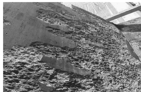
Fig.10. Spalling of Concrete Wall after The Fire
