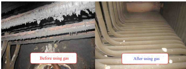
Fig. 1. Tube inside boiler before and after using gas
