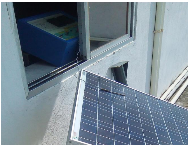
Fig: 1-2 Temperature of the solar panel can be measured by RTD
