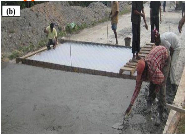
Fig. 3 (a) Casting of the PCCBP and (b) Laying of plastic cell formwork for next PCCBP section.
