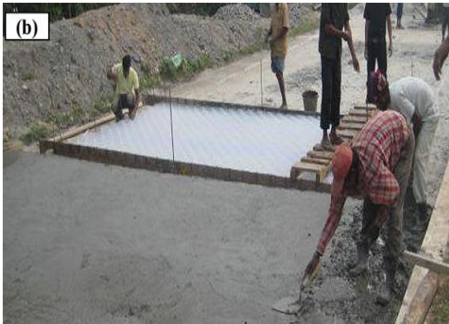
Fig. 3 (a) Casting of the PCCBP and (b) Laying of plastic cell formwork for next PCCBP section.
