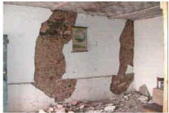
(b) Severely damaged stone masonry low-cost school buildings in 2006 Sikkim Earthquake
