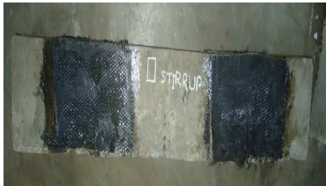
Fig. 4.4 Failure of Beam N-SB1
