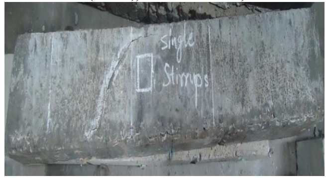
Fig. 4.3 Failure of Beam H-CB1
