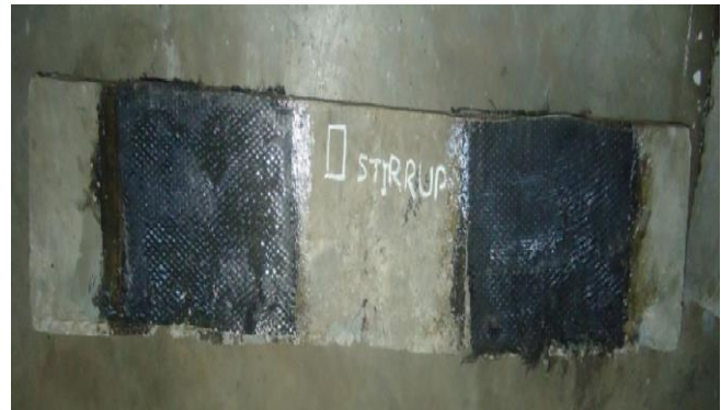
Fig. 4.4 Failure of Beam N-SB1
