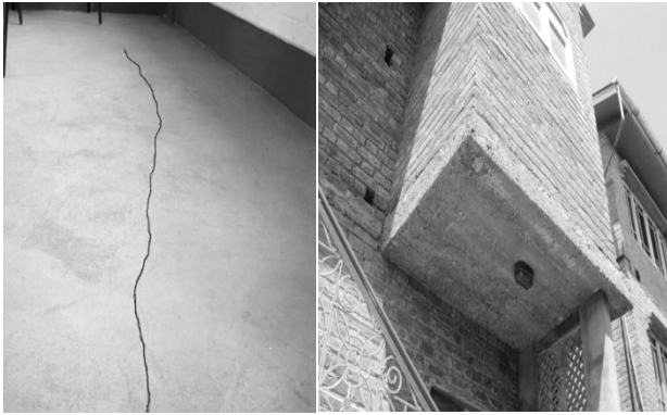
A. Cracks in Slab B. Overhead Projections
