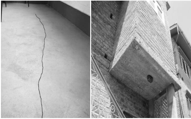
A. Cracks in Slab B. Overhead Projections
