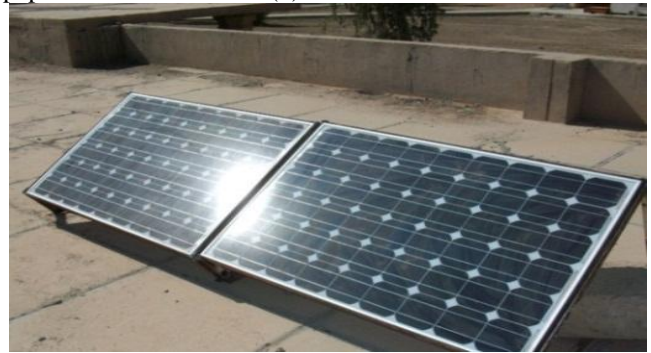
Fig. 6. The solar panels that used in the work
