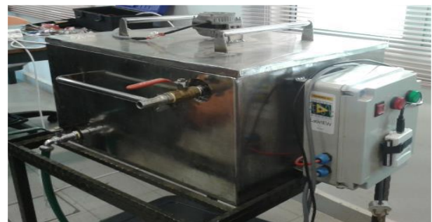
Figure 2: Water Tank System
