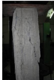
Fig. 5: Failure Pattern of Column Element CC
