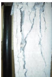
Fig. 3: Failure Pattern of Column Element CA
