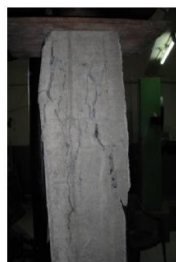
Fig. 5: Failure Pattern of Column Element CC
