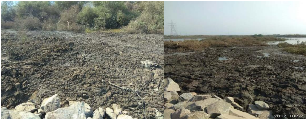
Fig.6: oozing/displacement of clay after end on dumping of blasted rocks (Source CIDCO)
